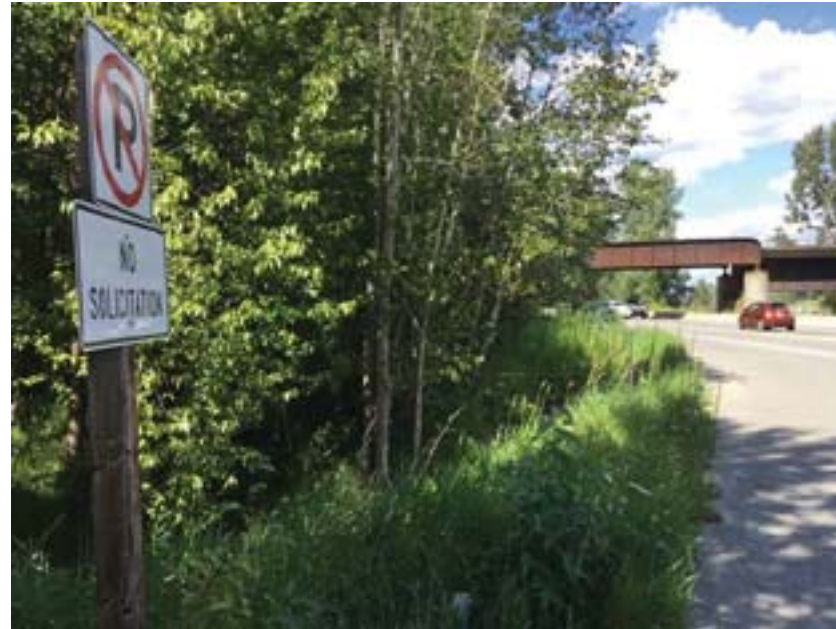
From turn off facing north with sign for orientation, culvert is central in frame.
